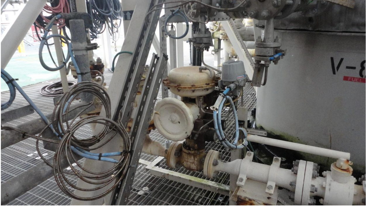
SPDC Equipment/ Control Room 7
