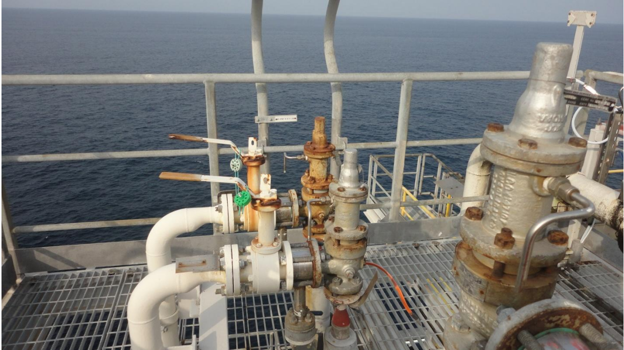
SPDC Equipment/ Control Room 4
