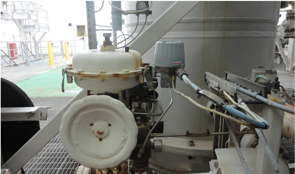
SPDC Equipment/ Control Room 9
