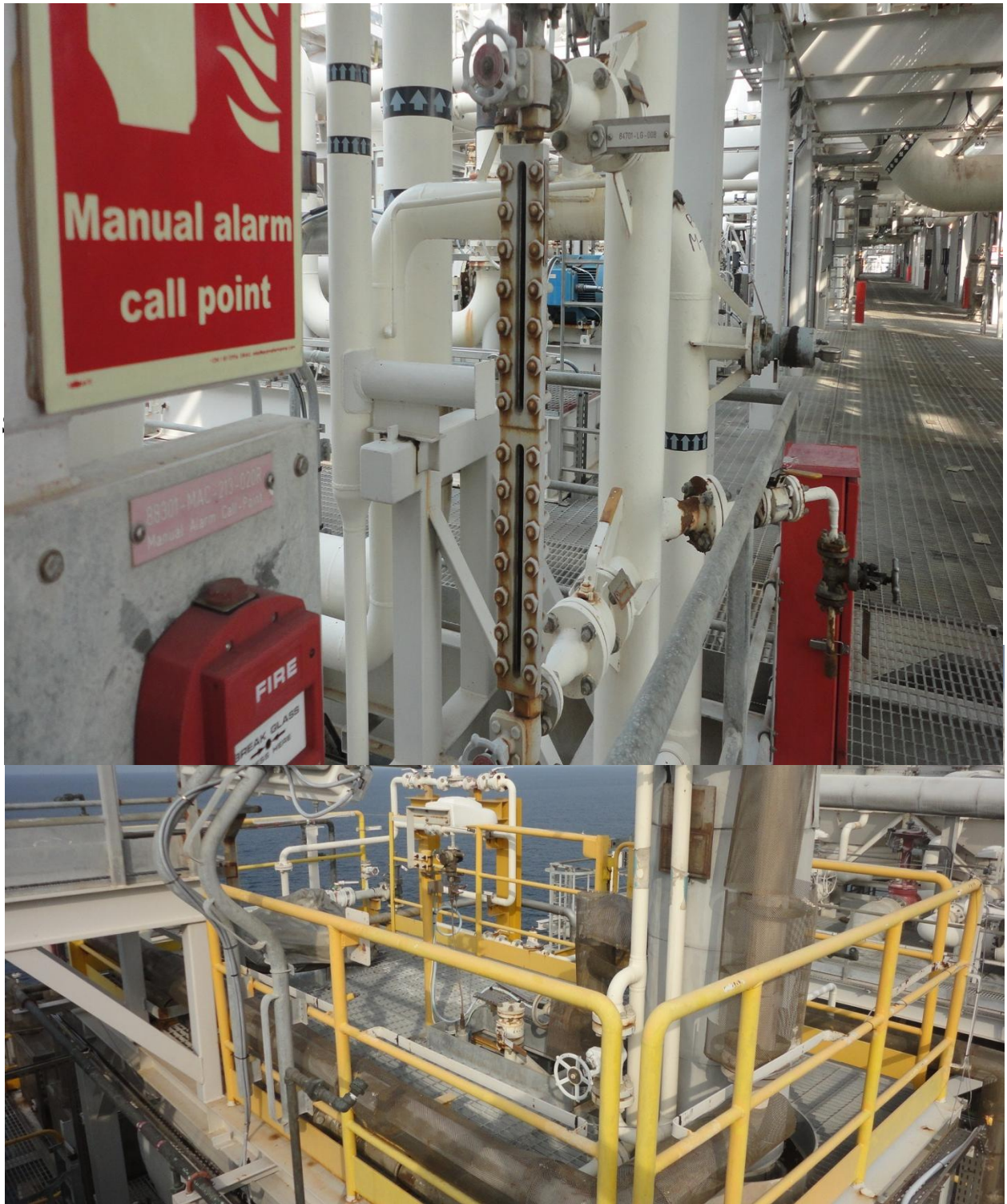
SPDC Equipment/ Control Room 3
