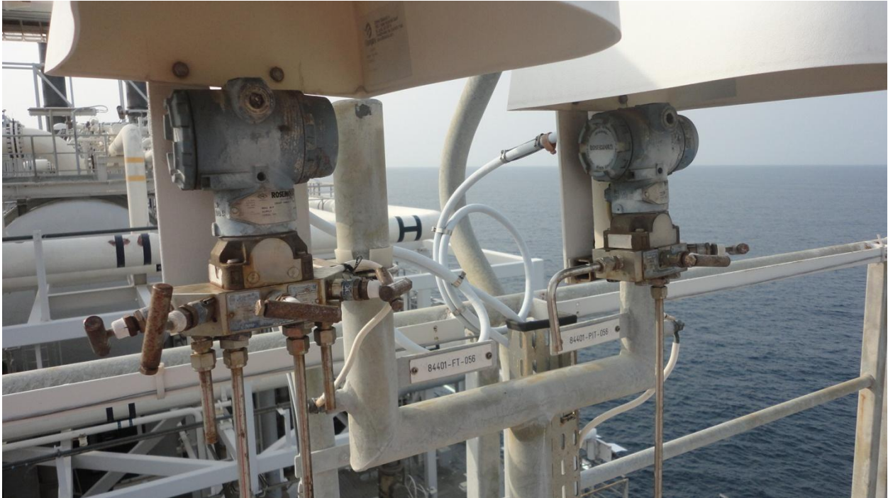
SPDC Equipment/ Control Room 5
