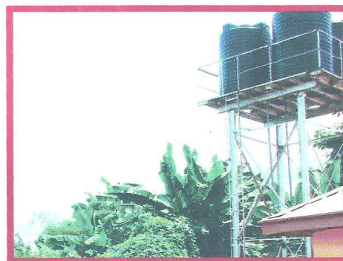
Water horehole provided by an individual in Omasi Health Centre Ayamelum L.g.A Anambra State
