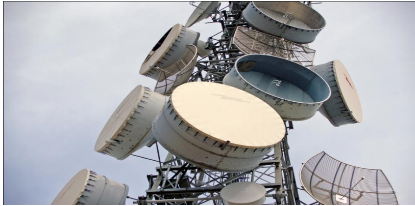
Figure 2.4: Typical Microwave mounted on a telecommunication tower (Wikipedia, n.d)
