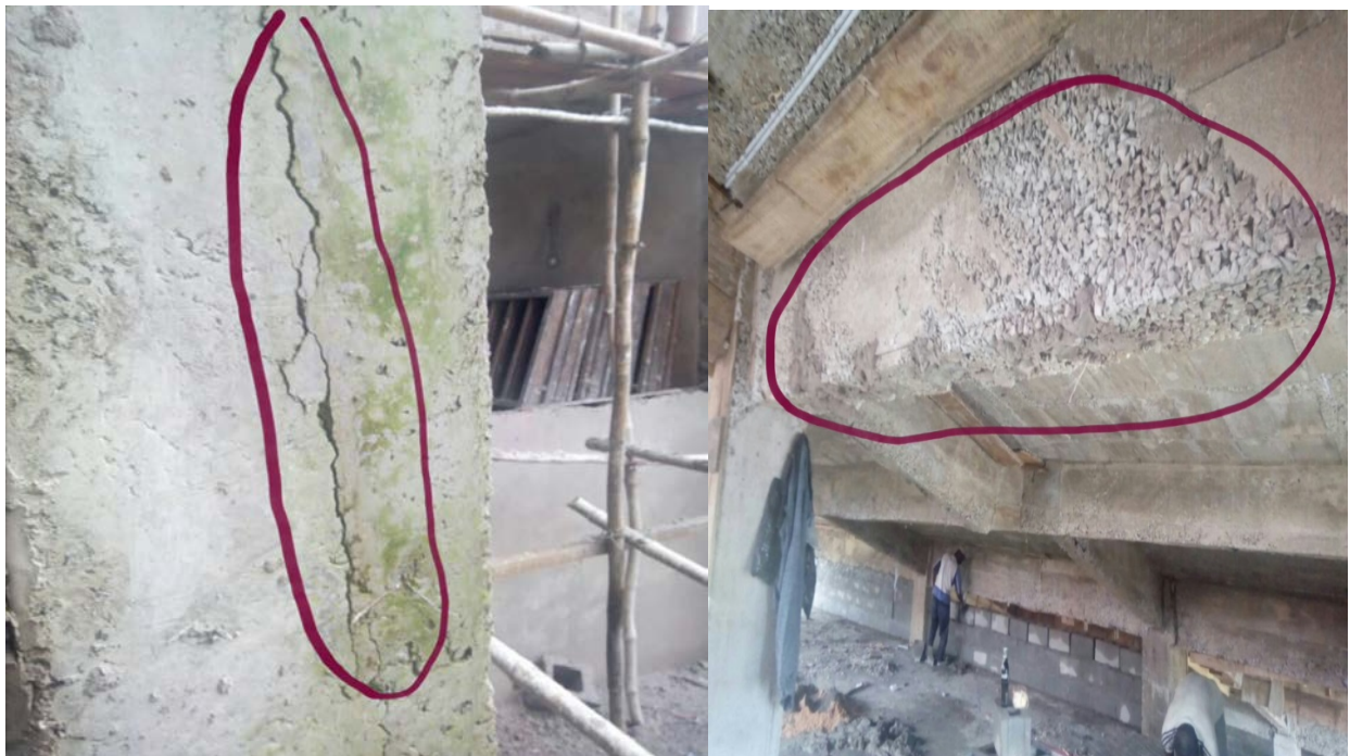
Plate VII: Major crack in a column of an ongoing project
