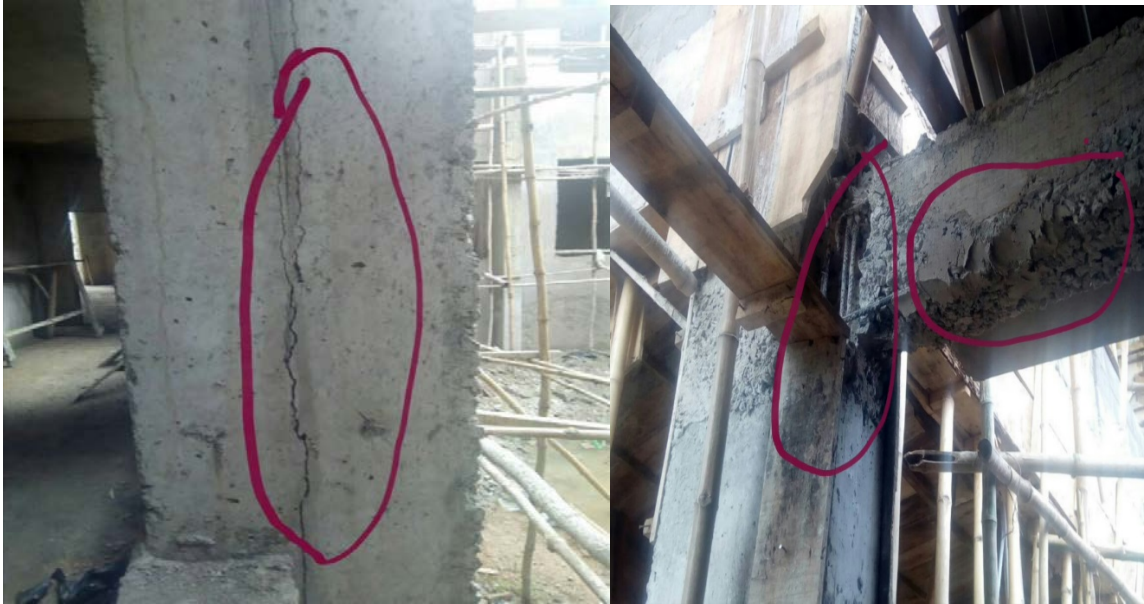
Plate V: Major crack in a column of an ongoing project
