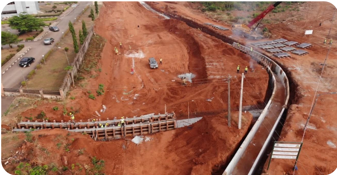
Fig. 4.21 Ekwueme Square/Fed. High Court Awka Erosion Site, 2019 During NEWMAP Intervention
