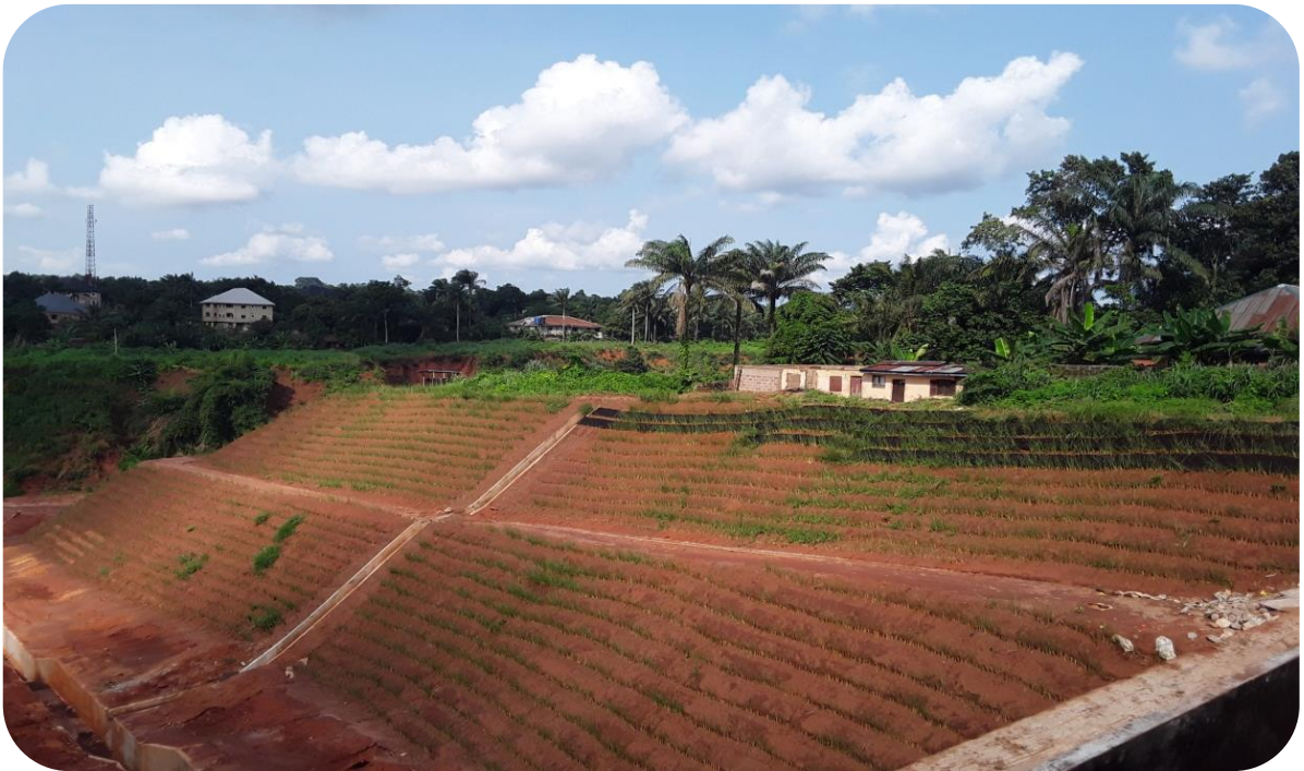
Fig. 4.19 Nnewichi Erosion Site, 2019 During NEWMAP Intervention
