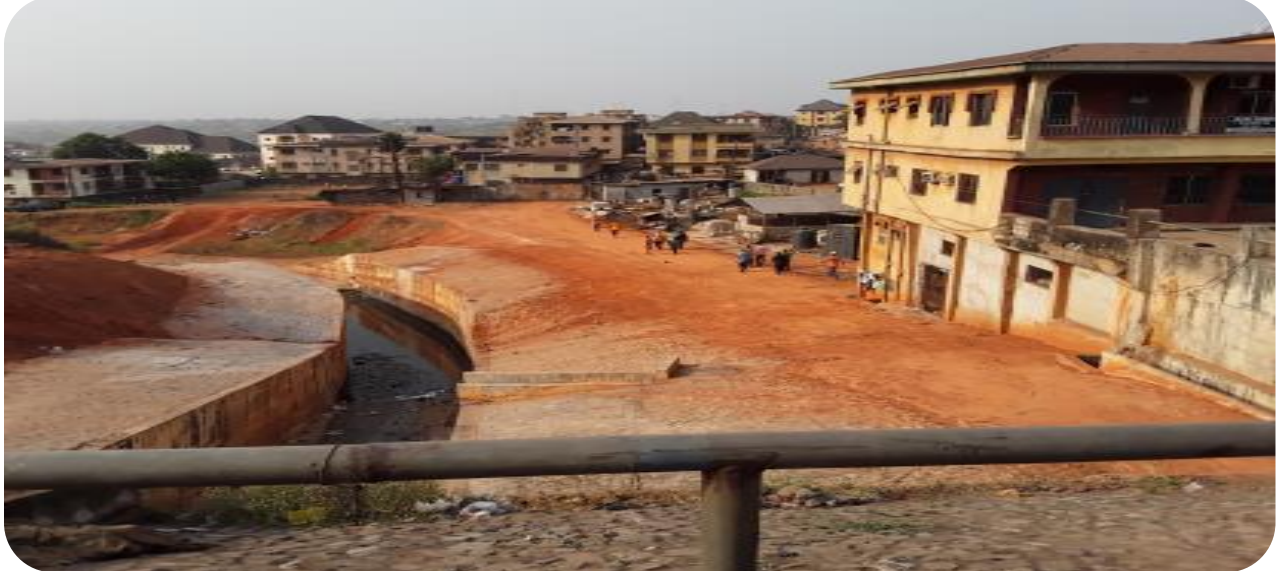
Fig 4.17 New Heritage Omagba/Onitsha Erosion Site, 2019 During NEWMAP Intervention
