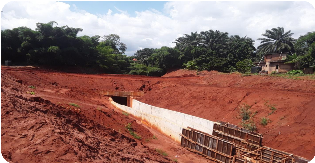
Fig. 4.13 Re-awarded Abagana Erosion Site, 2019 during NEWMAP Intervention
