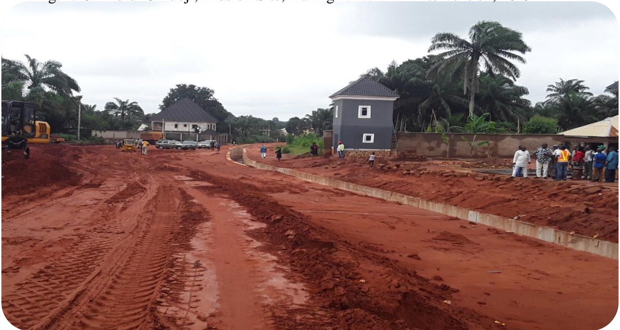
Fig. 4.25 Abidi Umuoji, Erosion Site, During NEWMAP Intervention, 2019
