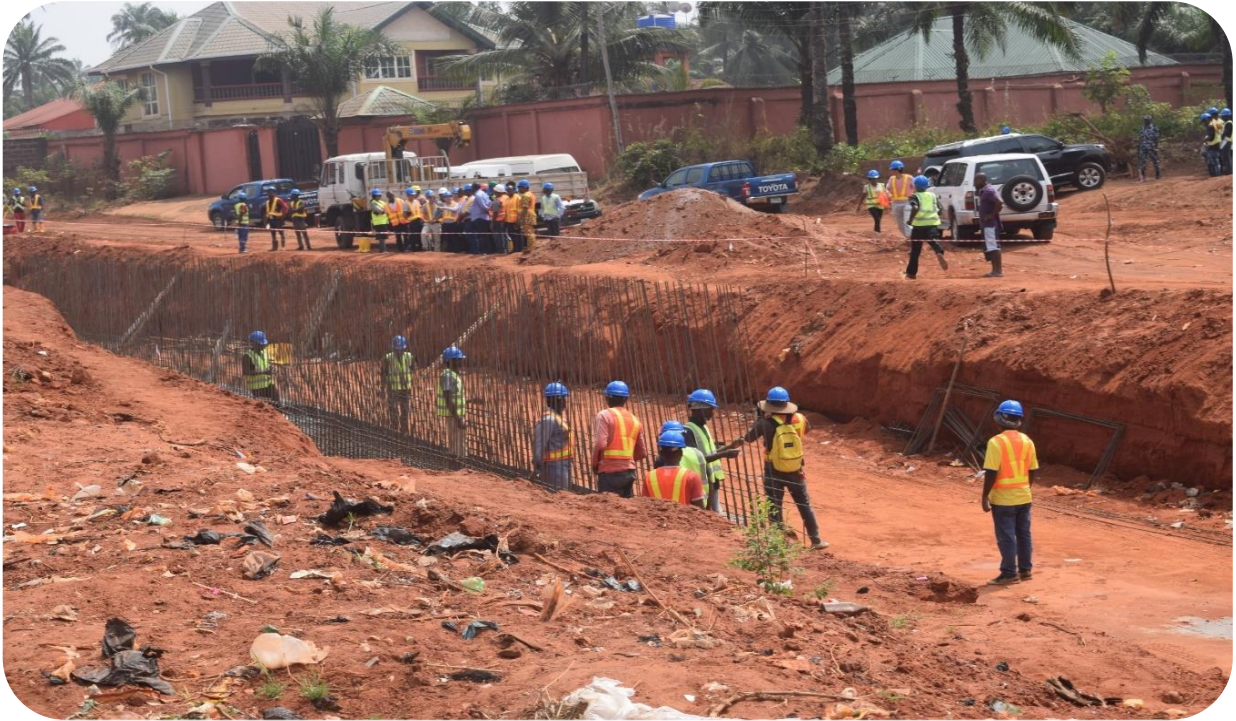
Fig. 4.24 Abidi Umuoji Erosion Site, 2013 Before NEWMAP Intervention
