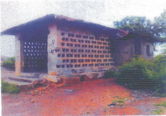
Colonial Mining Equipment House at Ameka Ezza in Ezza South Local Government Area, Ebonyi State.
