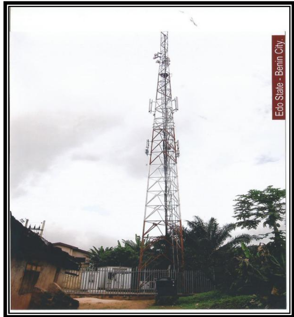
Figure 27: Isumwa Quarter; Mrs. Esohe-Esosa Erharuvi's Compound (2 meters to the house and 25 meters in height)
