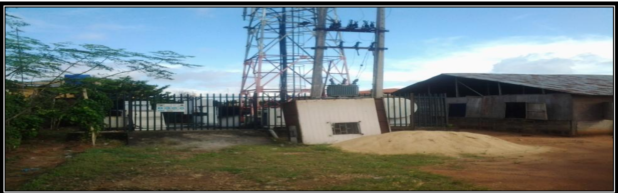
Figure 19: Amb. Leo Okogwu Quarters; Amaechi Agusi's compound (3 meters to houses, 25 meters in height)
