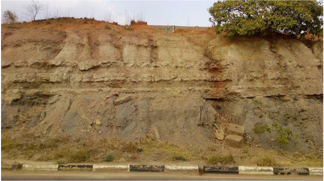
Fig. 4.20b: Photograph of the Outcrop Section at Independence Layout, Akagbe-Ugwu along Enugu to Port Harcourt, Exp. Way, Enugu State
