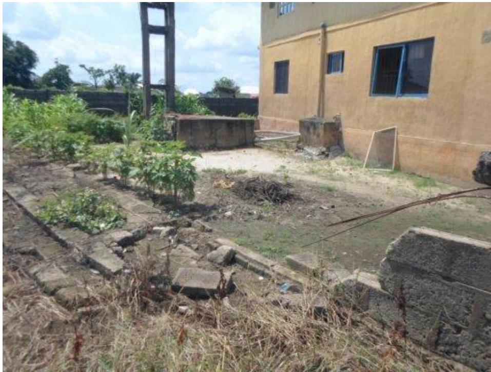
Plate 5.9 A fence pulled by flood water
