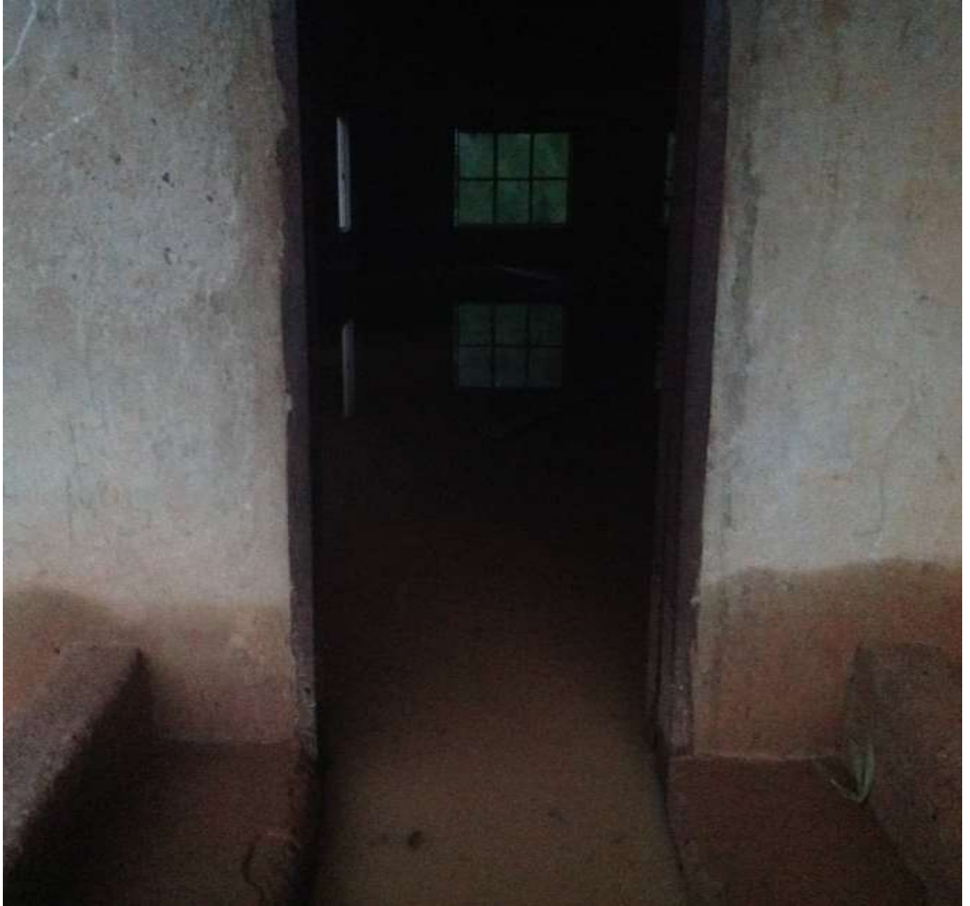
Plate 5.7: A building flood in Enugu South LGA
