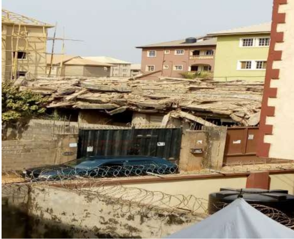
Plate 5.6: A collapsed building in Enugu Metropolis that resulted after rainfall
