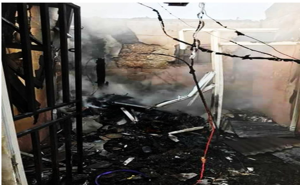
Plate A3b: showing one of the shops that was consumed by fire Source: ( https://www.nationalhelm.co/2018/01/tetlow-plaza-owerri-fire-goods-peoperties-destroyed-photos.html January 25, 2018)
