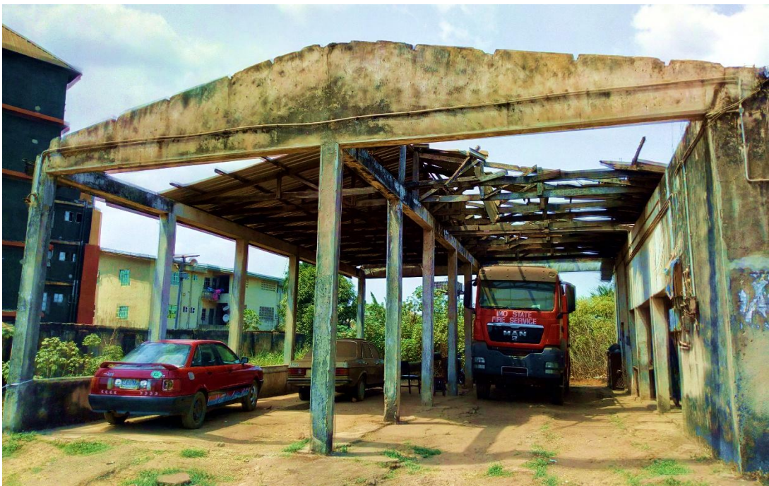
Plate B2: showing the level of degradation
