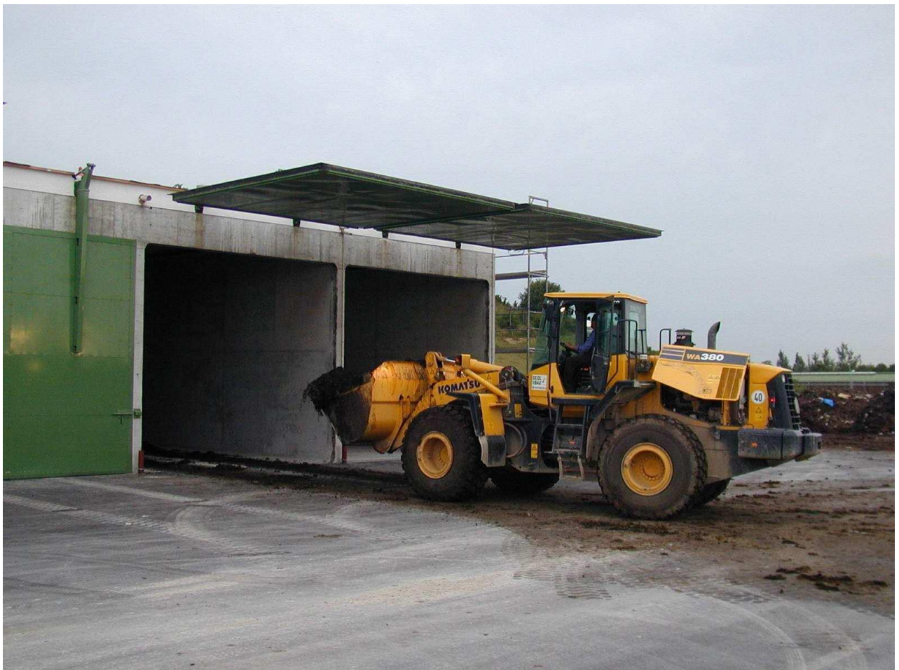
Figure 2.6: Garage-type batch digester, loaded by a loader (BEKON, 2004)
